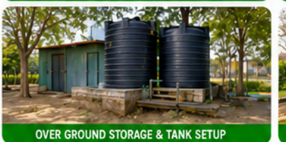
OVER GROUND STORAGE & TANK SETUP
