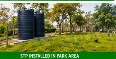
STP INSTALLED IN PARK AREA
