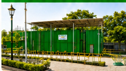
200 KLD DSTP INSTALLED AT SHUBROTO PARK
