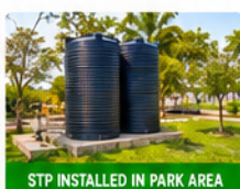
STP INSTALLED IN PARK AREA
